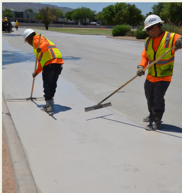
Figure 4.7. Workers applying a cool surface coating to streets in the City of Phoenix as part of a pilot project being evaluated by Arizona State University (City of Phoenix)
